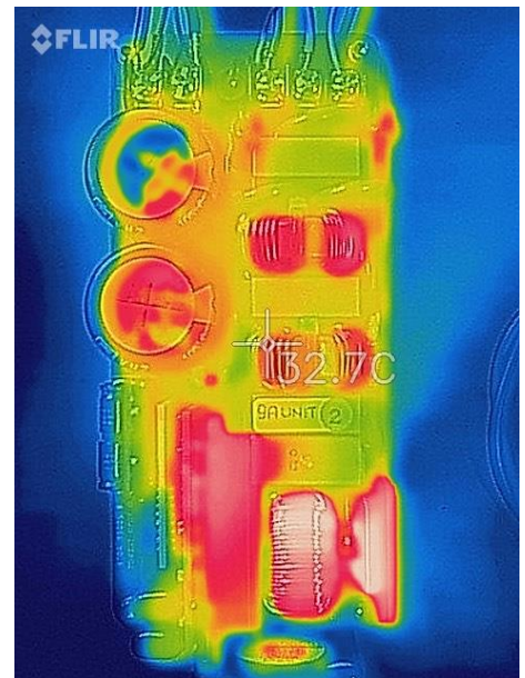
Figure 47: Vertical top-side thermal image
